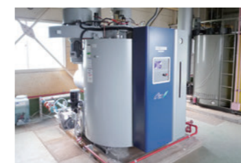
Boilers were upgraded to high-efficiency products
